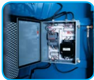
BE-TS Control Panel
